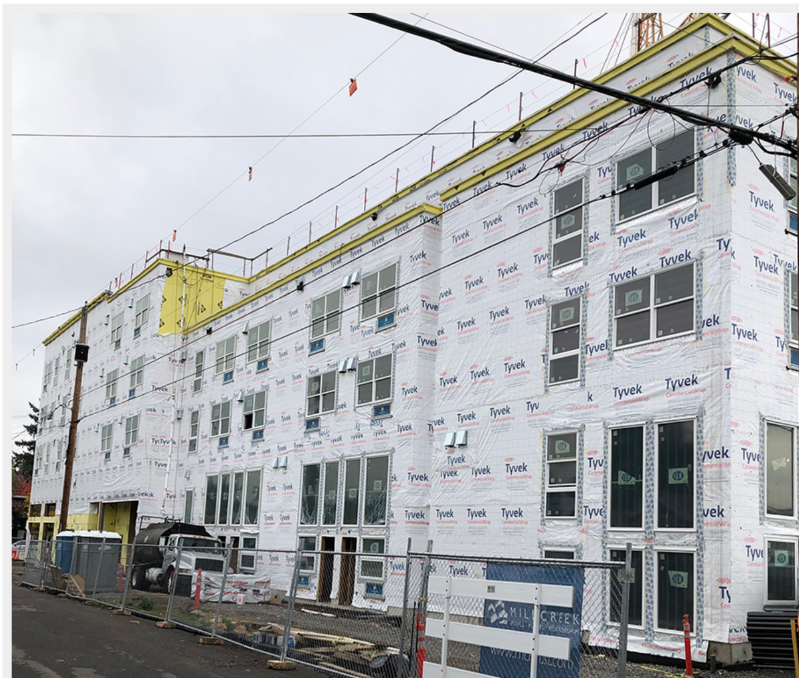
Construction of Modera Woodstock is scheduled to finish this fall. (courtesy of Leeb Architects)
